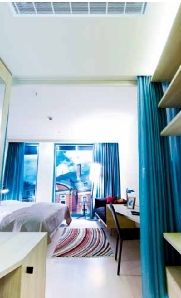
In the entrance lobbies of the rooms, active chilled beams are installed in the ceiling void. The supply air is introduced to the room through louvred grilles and removed again from the bathroom via disc valves.
